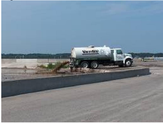
Septic hauler discharging at the off-loading site
